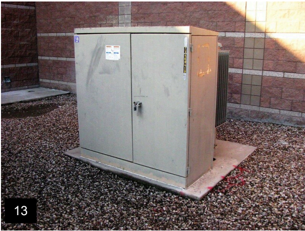
13 Typical APS transformer
