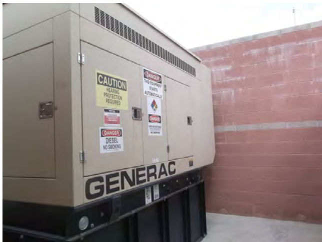
Emergency generator with AST
