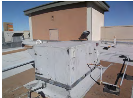
PHOTO #12 HVAC EQUIPMENT
