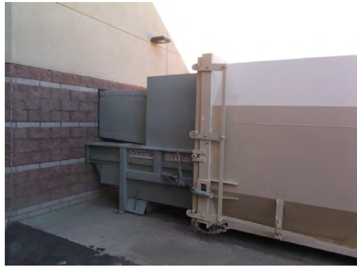
PHOTO HYDRAULIC TRASH COMPACTOR #26
