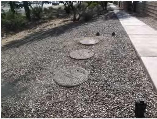
PHOTO GREASE TRAP #25
