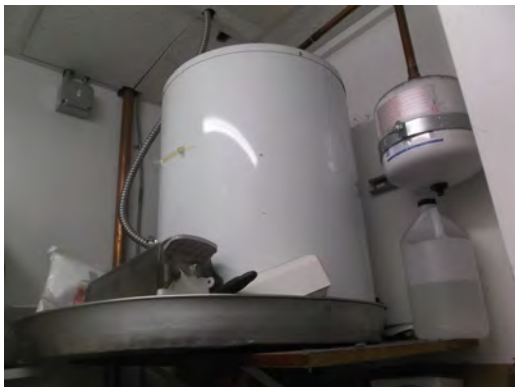
PHOTO #11 WATER HEATER
