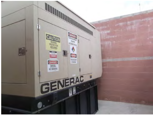
PHOTO #31 EMERGENCY GENERATOR WITH AST
