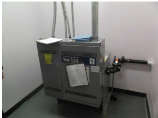
PHOTO ELEVATOR EQUIPMENT #30
