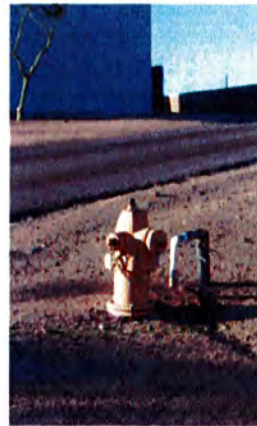
Hydrant north of Transfer Building
