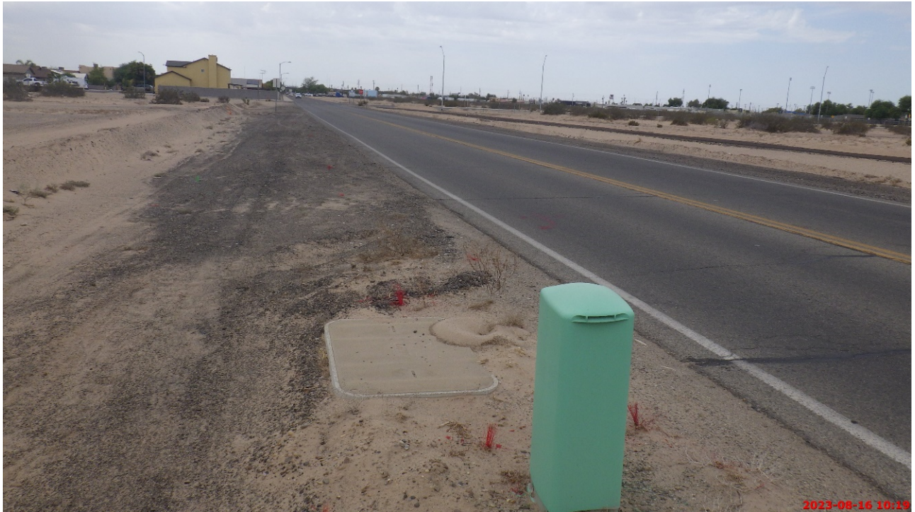
View from the western project limits (within City of San Luis Easement on ASLD Land) looking south towards electrical pedestal and associated pull box.
