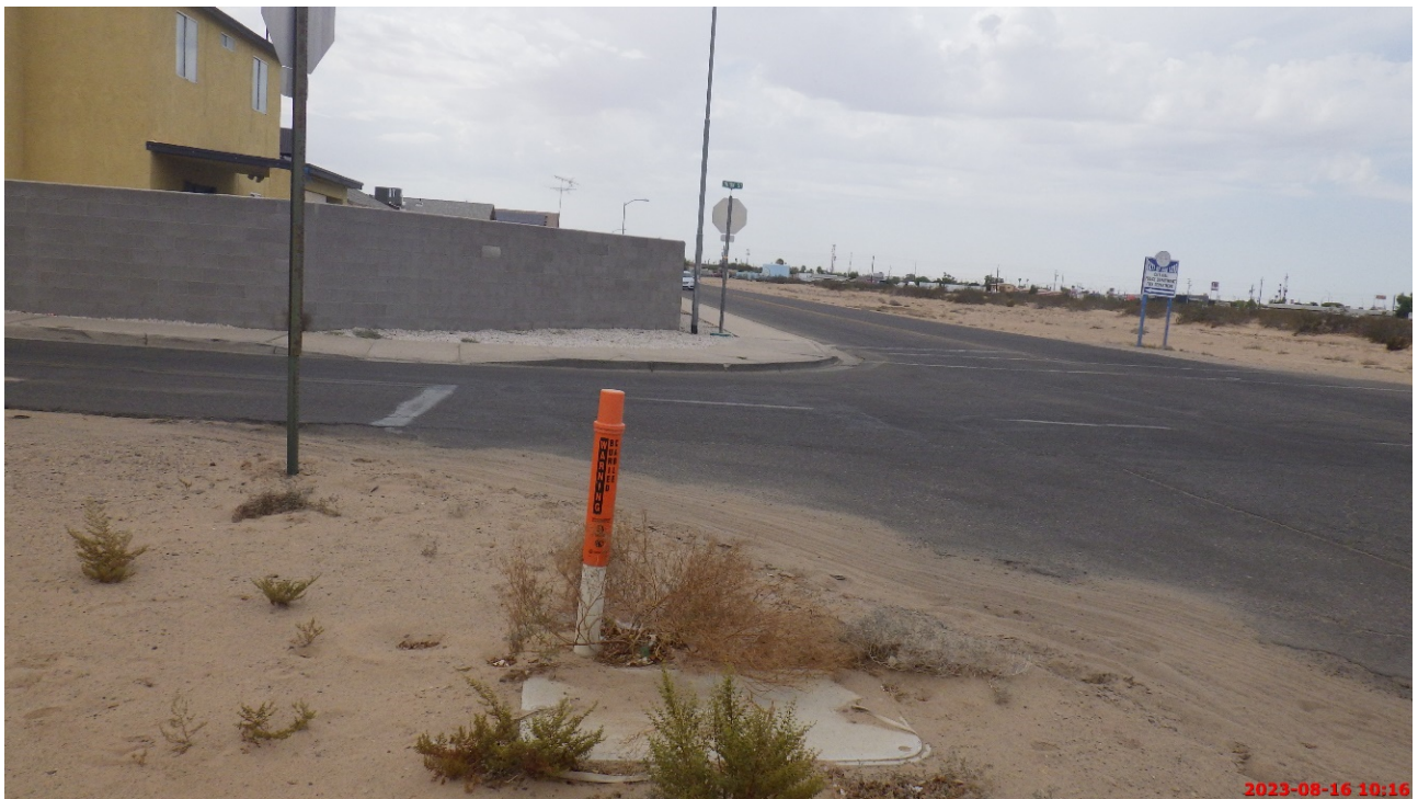
View from the southwestern corner of the project limits looking south toward cable and associated pull box.
