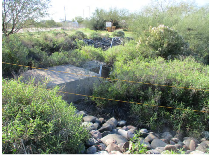
Photograph 14 – A view of the culvert exit at the north end of the main wash, looking southeast.
