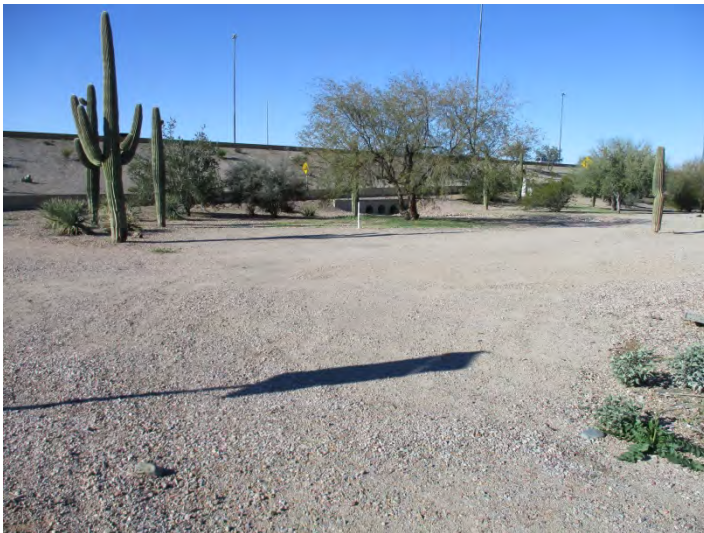
Photograph 27 – A view of the south adjoining Pima Freeway segment of State Route 101 (Loop 101), looking southwest, showing the box culvert.
