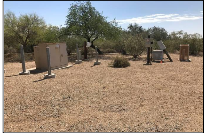
Picture 8 - The APS pad-mounted transformer and utility boxes just east of the lift enclosure.
