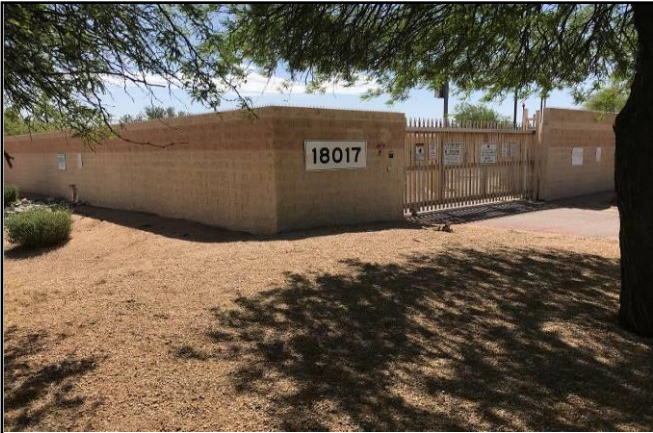
Picture 6 - The City of Phoenix lift station enclosure on the southwest portion of the Property.
