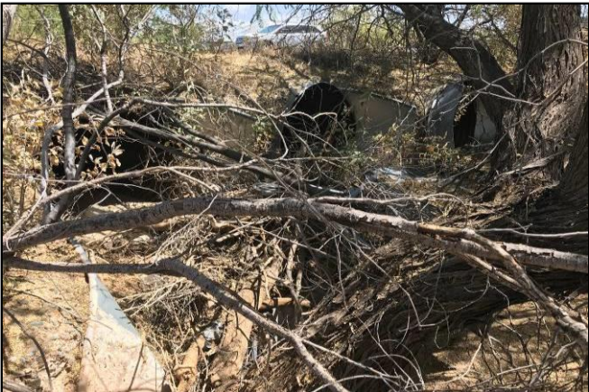
Picture 4 - The three culverts that channel stormwater from north of Mayo Boulevard into the wash on the Property.
