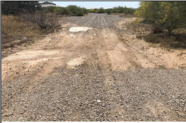
Picture 5 - The gutter drain on the gravel driveway on the south Property boundary that channeled stormwater from the wash off the Property.
