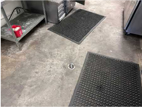
Photo #31 View of typical interior floor drain located in the kitchen of the Shipwrecked Pirate Bar and Grill.
