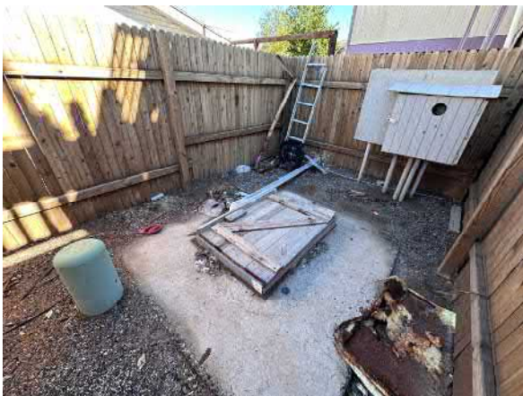
Photo #29 View of the septic pump located south of the restroom and shower building on the central portion of the site.
