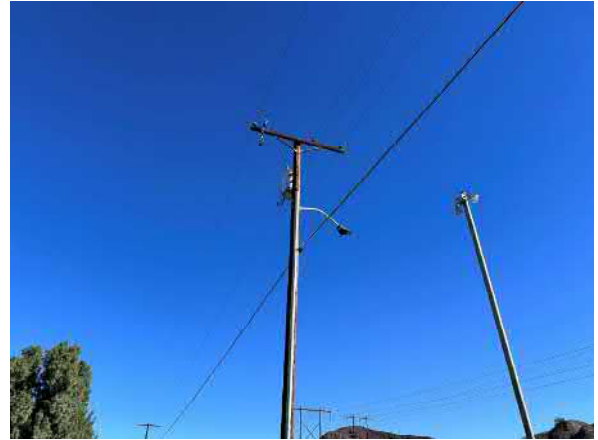
Photo #32 View of typical pole-mounted transformer located on the eastern site boundary.
