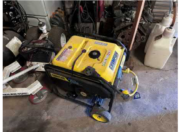
Photo #14 View of the 6520-Watt portable generator located inside the eastern storage building.
