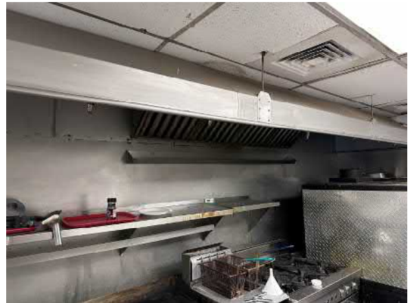
Photo #16 View of the ventilation hood located in the kitchen of the Shipwrecked Pirate Bar and Grill.
