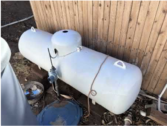
Photo #19 View of typical 250-gallon propane tank.
