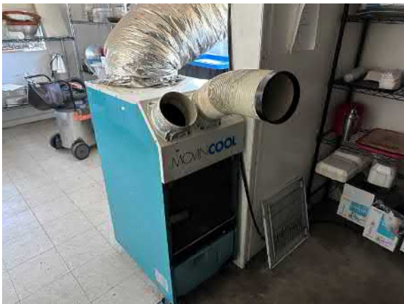
Photo #17 View of cooling system located inside the kitchen of the Shipwrecked Pirate Bar and Grill.
