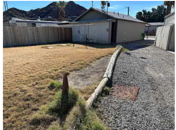
Photo #28 View of the central septic holding tanks.
