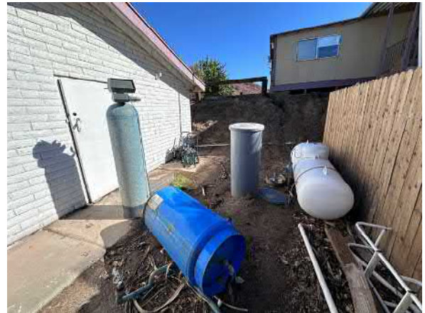
Photo #26 View of typical 250-gallon empty water softener tanks located on the central portion of the site.
