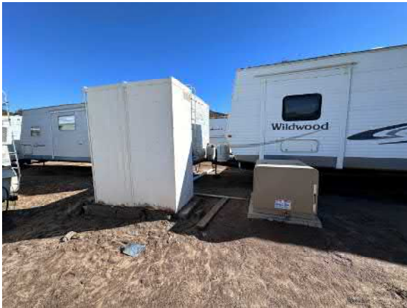
Photo #33 View of the pad-mounted transformer located on the central portion of the site.
