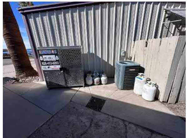
Photo #18 View of typical 20-pound propane tanks located on the eastern portion of the Shipwrecked Pirate Bar and Grill.
