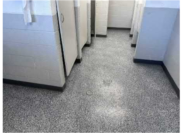
Photo #26 View of typical interior floor drain located throughout the site.
