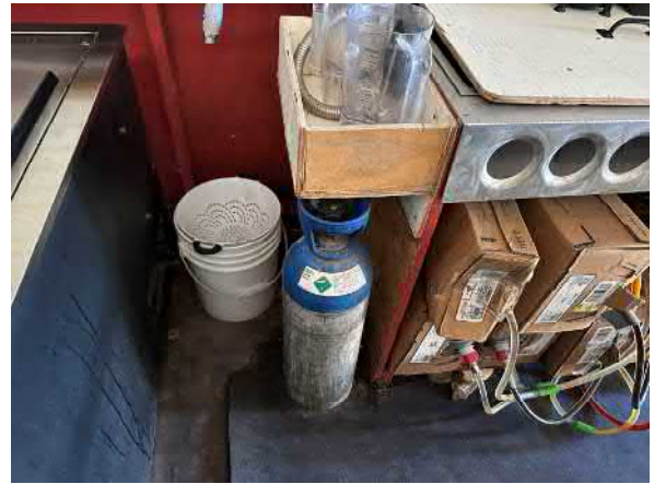
Photo #16 View of typical compressed CO 2 tank located throughout the bar and kitchen areas of the site.
