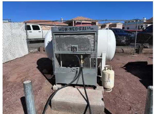
Photo #18 View of the propane tank filling station located on the western portion of the site.
