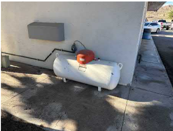
Photo #17 View of typical propane tank used throughout the site.
