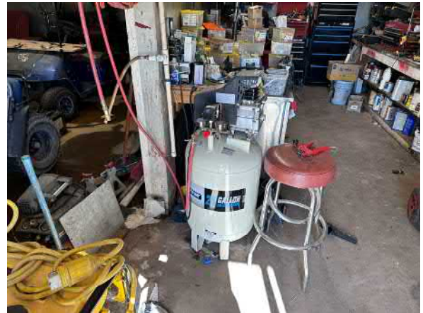
Photo #14 View of typical air compressor, located inside the maintenance shop on the northern portion of the site.
