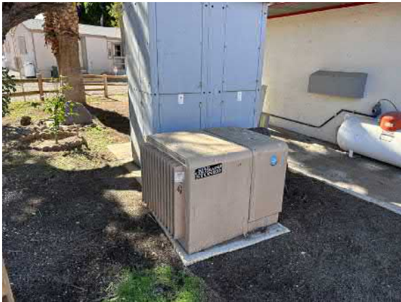
Photo #27 View of the pad-mounted transformer located on the northwestern portion of the site.
