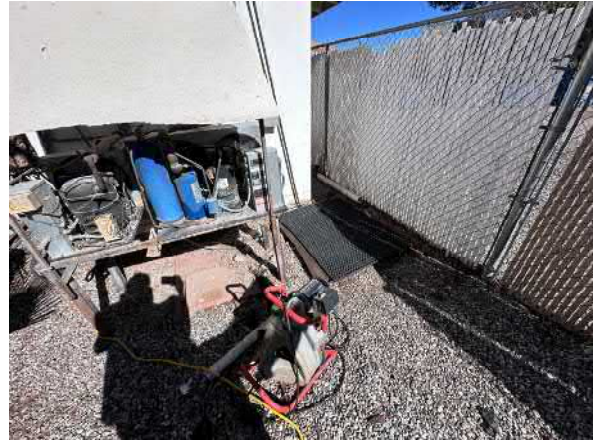
Photo #22 View of the one of the septic tank locations located on the western portion of the site.
