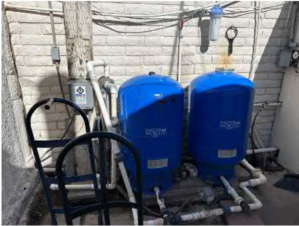
Photo #19 View of river water pressure tanks located on the western portion of the site.
