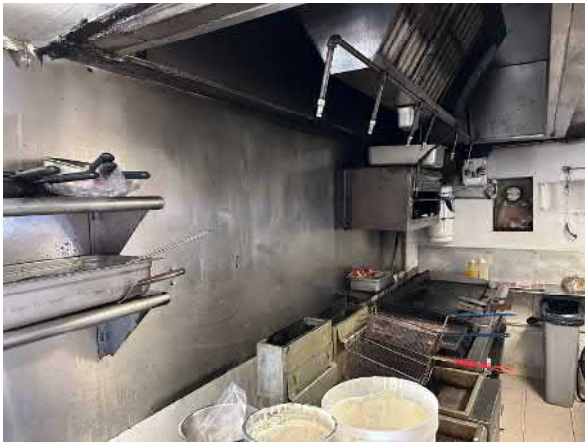
Photo #15 View of ventilation hood located in the kitchen on the western portion of the site.
