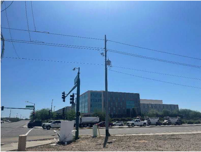
Photo No. 13: View of pole-mounted transformer located near the northeast corner of the Property; view to the east.
