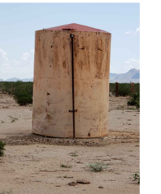
Existing Vertical Tank
