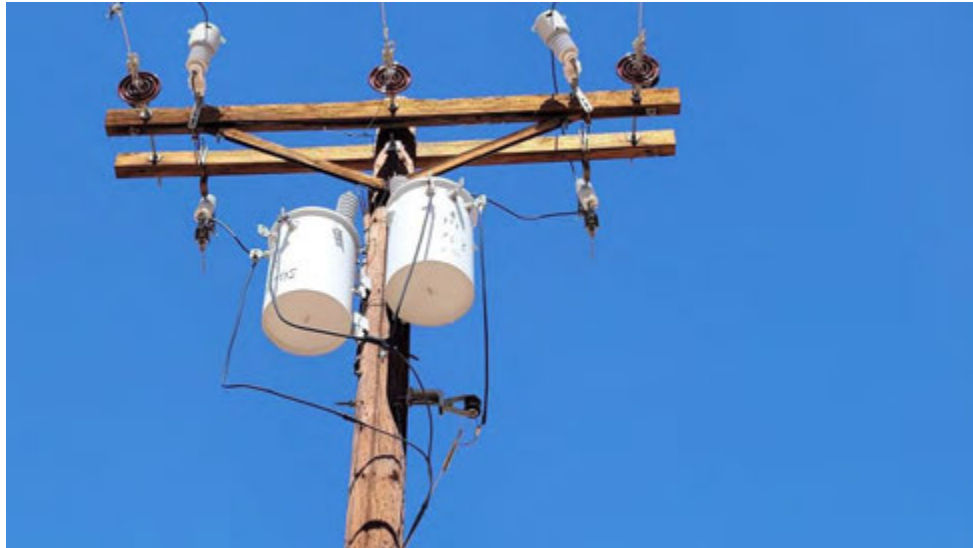
Photo 45: 7-9-22: Two pole-mounted transformers adjacent to the well. Both were in good condition with no evidence of leaks noted.
