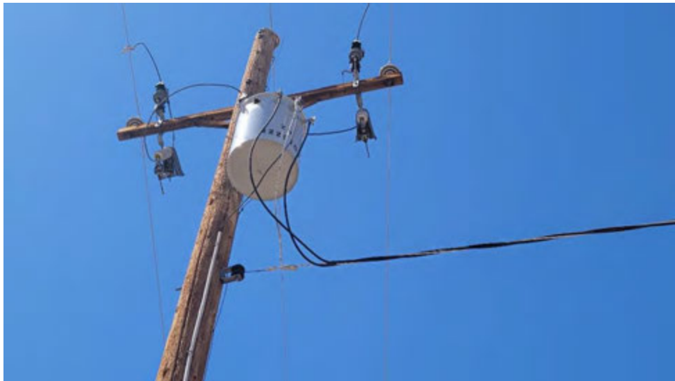
Photo 8: 6-16-22: Pole- mounted transformer on westernmost power pole. No evidence of staining or spills noted.
