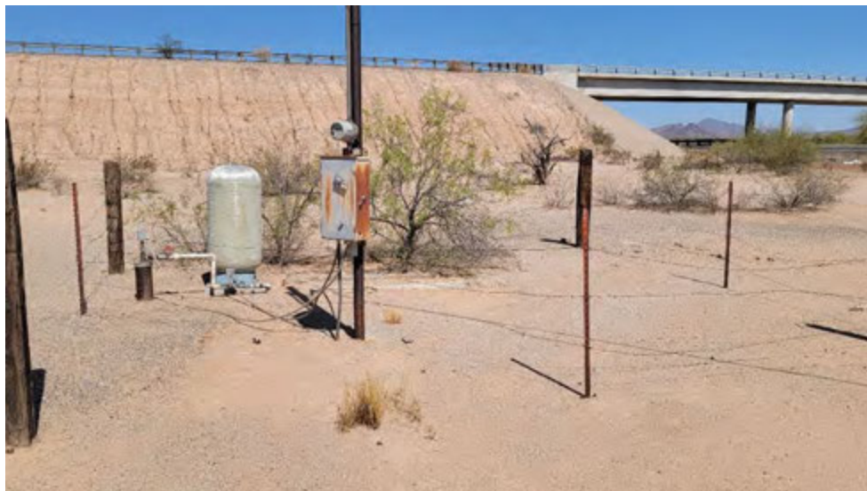
Photo 44: 7-9-22: Active well located adjacent to I-10 and Sore Finger Road in southeast segment of Subject Property. This ASLD well reportedly supplies water to the livestock drinker, and the corral.
