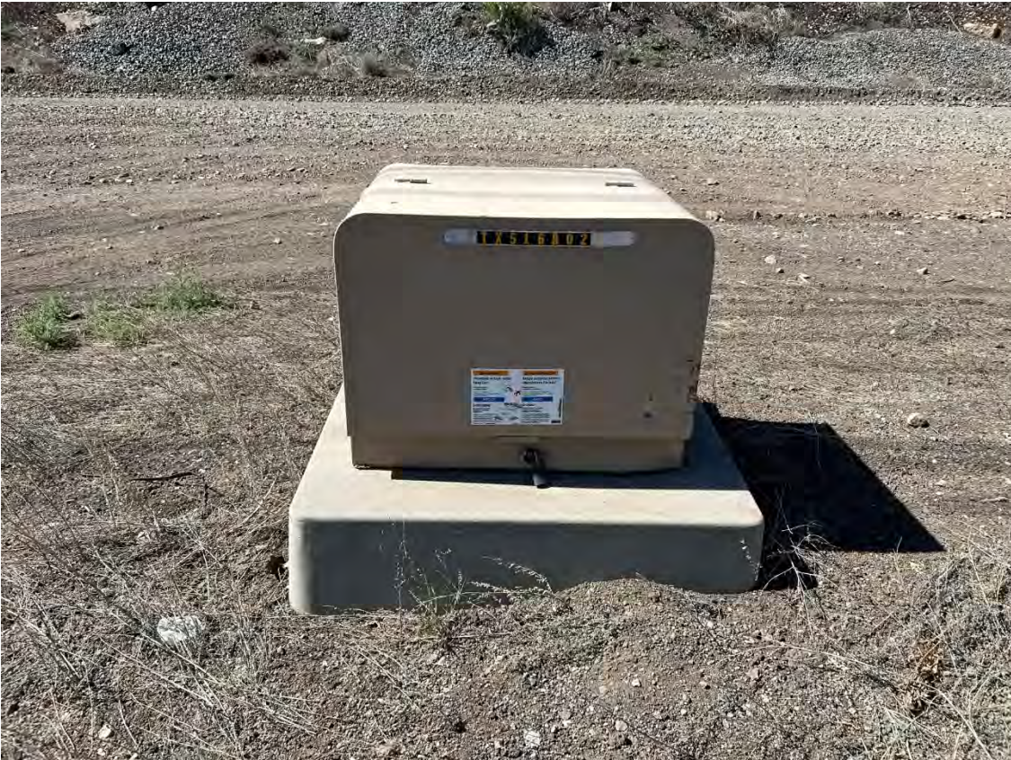
Photo 7 Transformer (1 of 3) along southern edge of Route 66.
