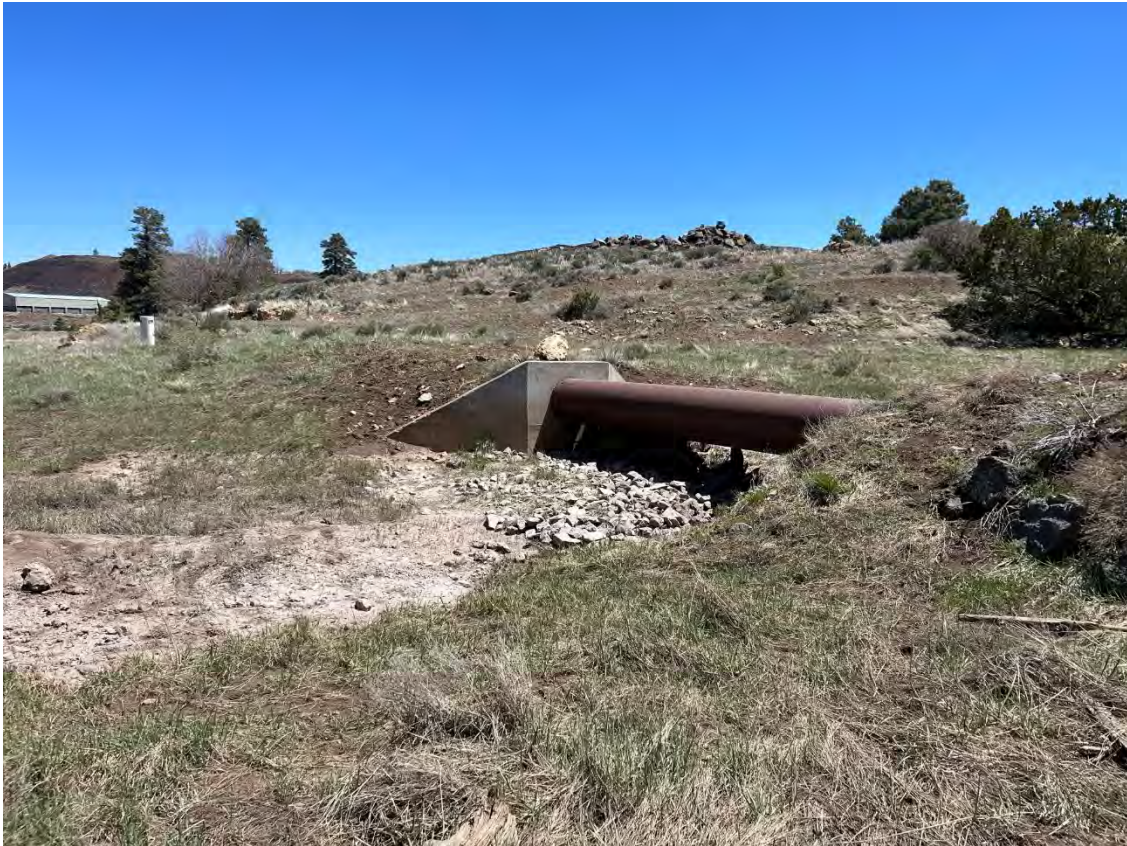
Photo 21 View of sewer line running south to north through the Subject Property.
