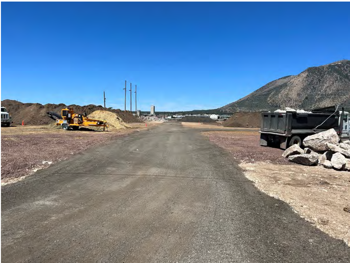
Photo 16 West view into Restoration Soils yard in the eastern portion of the Subject Property.
