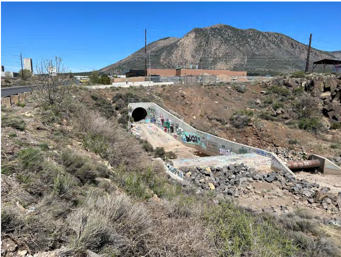
Photo 12 West view of Rio de Flag culvert opening east of the ADOT yard south entrance.
