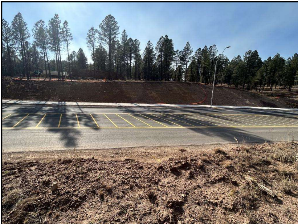
Photograph 8. South Fourth Street followed by construction activity west of the subject property.
