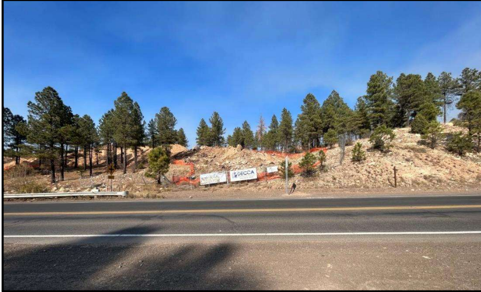
Photograph 5. East Butler Avenue followed by construction activity north of the subject property.
