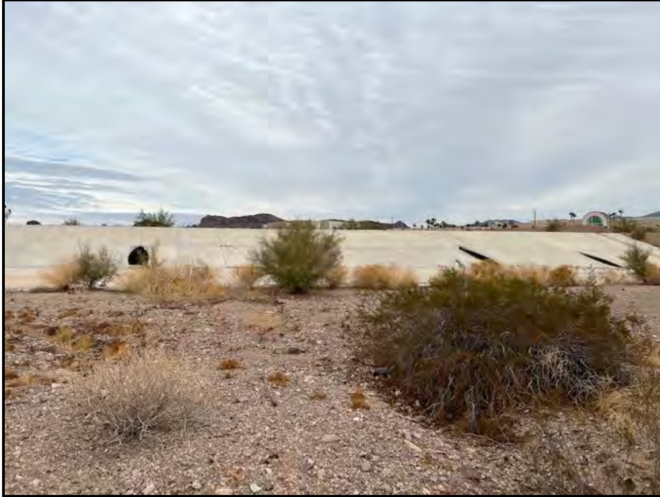
Photo 7: Concrete stormwater structure along Retail Center Boulevard within the subject property.
