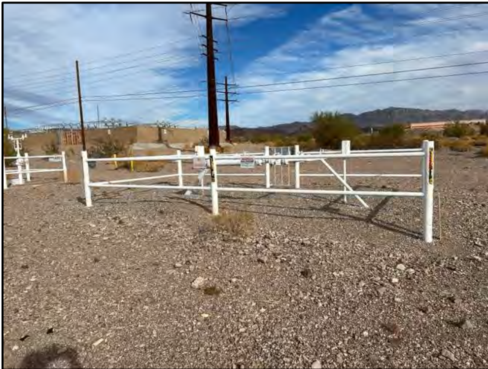
Photo 8: Pipeline valve sites observed in the southeastern corner of the subject property.
