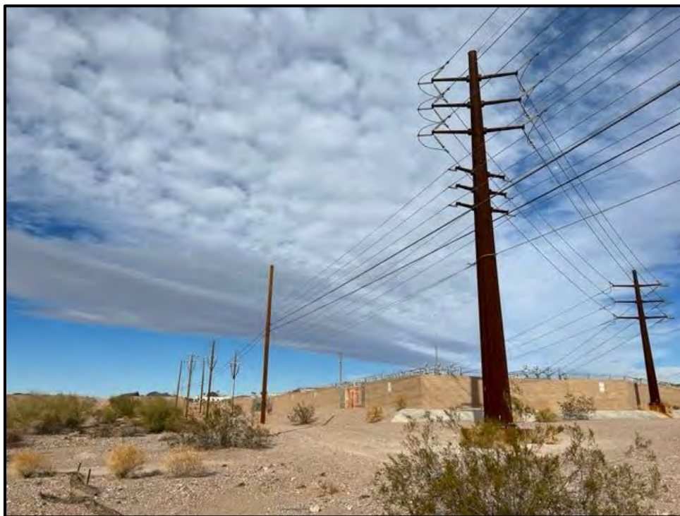
Photo 10: Transmission lines and substation adjoining the southeastern corner of the subject property.
