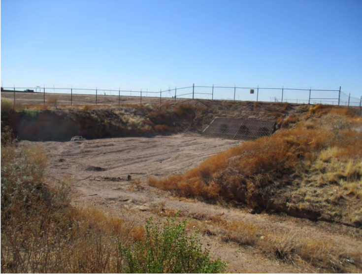
Photo 25 - View of the south of the two culverts through the Fannin-McFarland Aqueduct outside the subject property's west boundary.
