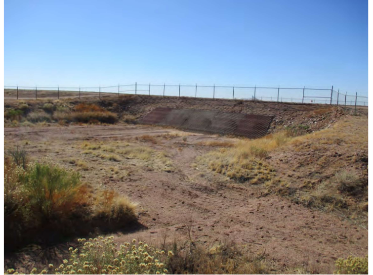
Photo 26 - View of the north of the two culverts through the aqueduct, looking southwest.
