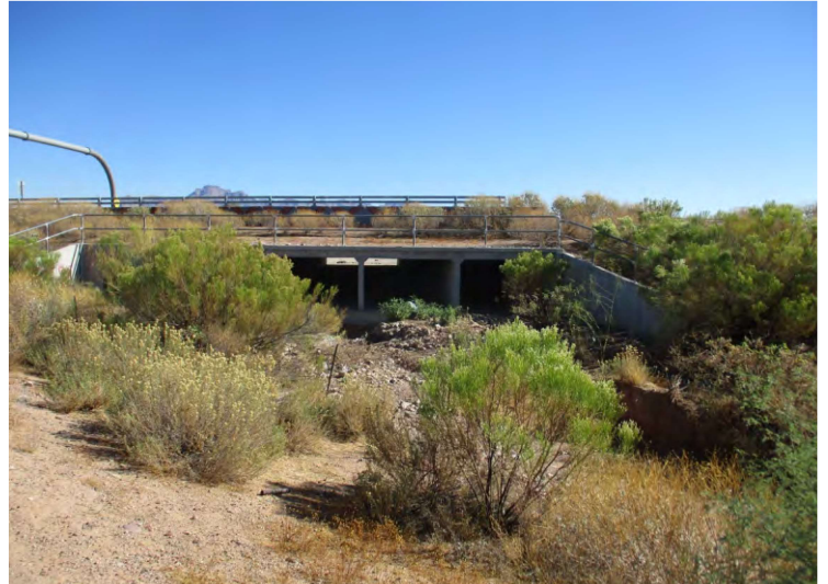
Photo 24 - View of the culvert under Meridian Road near the south corner of the subject property, looking east.
